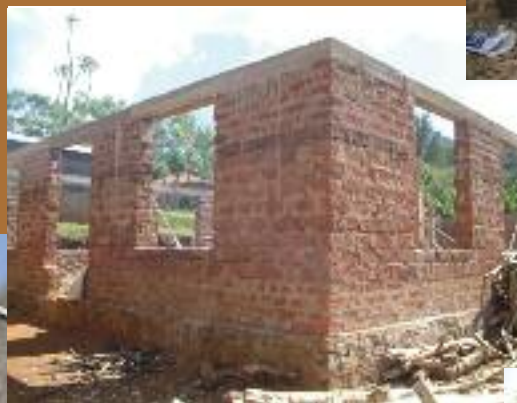
Shighatini Secondary School - ongoing construction to complete one classroom and finish a second
