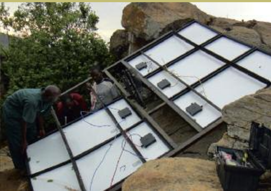
Storm damage to the solar power system at Kisima Camp
