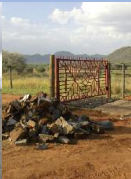
New heavy steel gates being put in place inbetween sections in the Rhino Sanctuary
