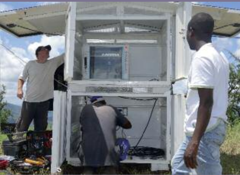
Phil King and his technician work with Fred Ayo to install the digital radio repeater on the top of Hafino Hill
