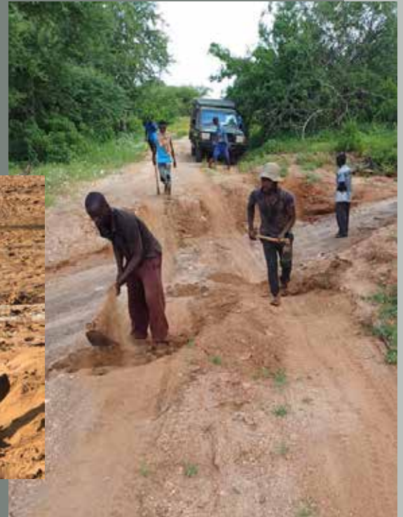
Teams of casuals bush-clearing and opening up the old roads and tracks
